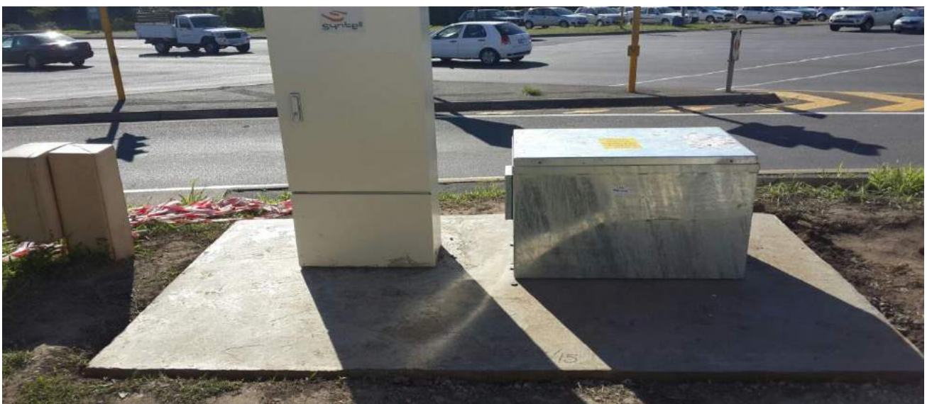
Figure – Installation of UPS equipment to power traffic signal equipment
