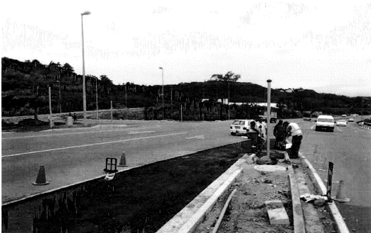
Figure – Installation of traffic signals at the intersection of Wyse Avenue and the N6 PUBLIC TRANSPORT (MUNICIPAL BUS SERVICE)
