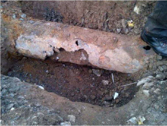
Above: Cambridge Street pipe crossing sinkhole
