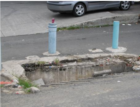
Above: Typical examples of current condition of Kerb Inlets
